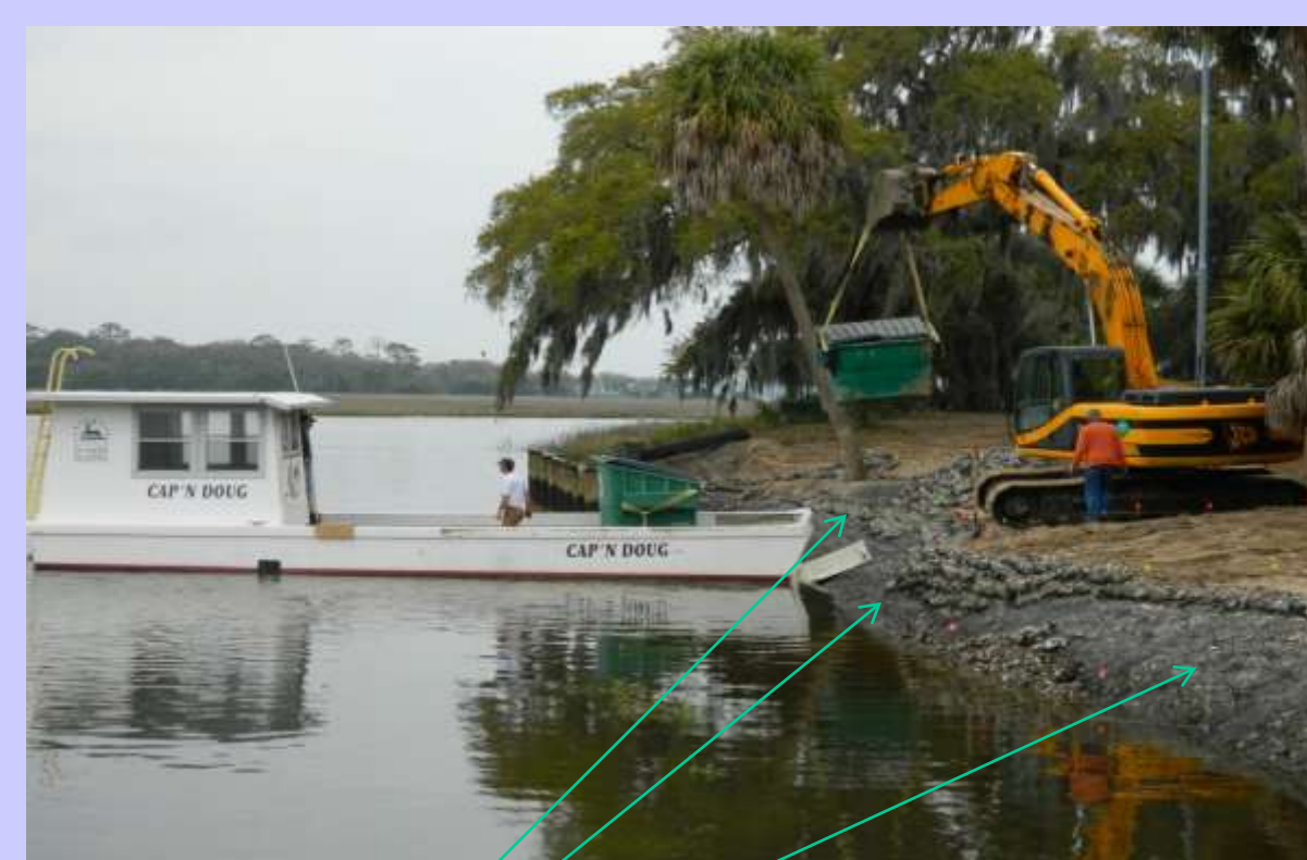
Figure 3. Photo of bank grading equipment unloading bagged shell and the geotextile fabric used in layering the oyster bags at the LSSI site.
